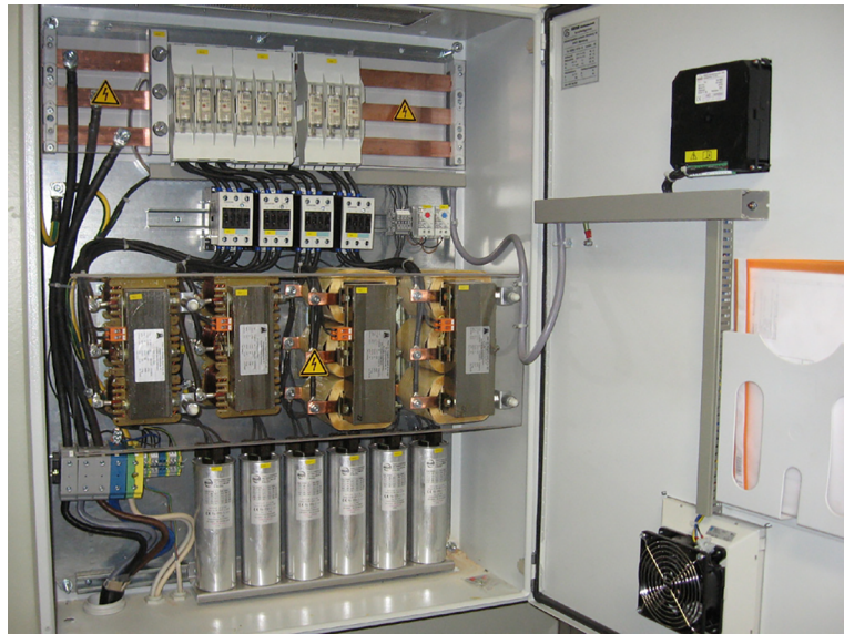
Figure 14: Example of a power factor correction unit used for plant-wide power factor correction. Notice the bank of capacitors located at the bottom of the unit.
