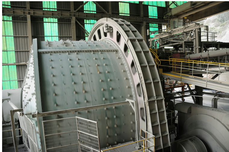
Figure 12: Any induction motor driving a large load such as the ball mill shown above requires a substantial amount of reactive power to operate. Using distributed power factor correction prevents the large reactive power requirement of the motor from affecting the power factor of the industrial application.
