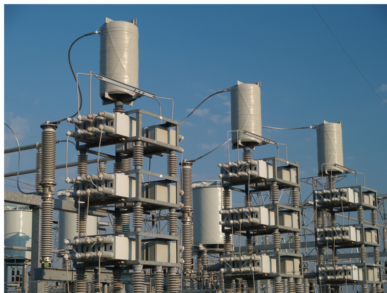
Figure 8: Bank of capacitors used for power factor correction.
